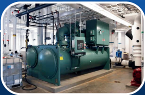
HVAC Performance Evaluation & Improvement
